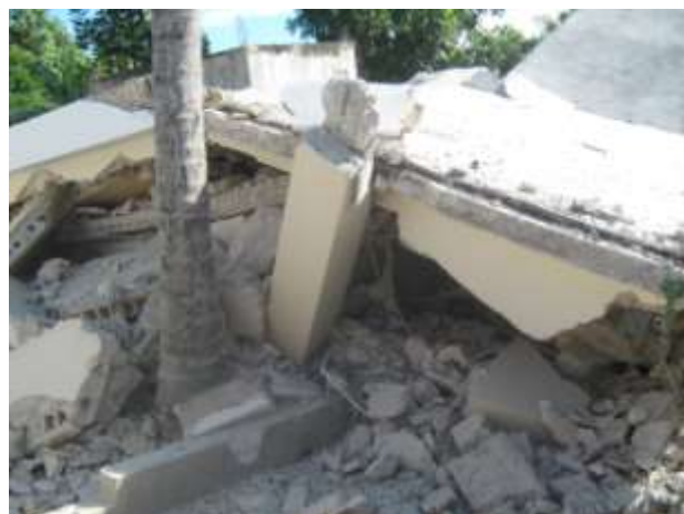
Pastor Osnel's House After
